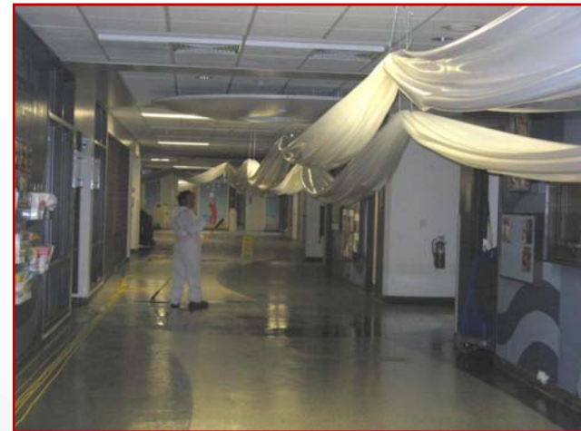
Cleaning up flood-damaged John Sealy Hospital
